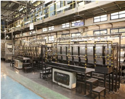
Chemical Weighing Station
